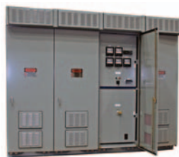
Medium voltage AC switchgear
