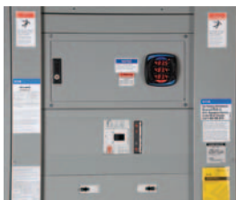
Custom Solar Switchboards
