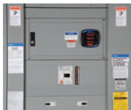
Custom Solar Switchboards
