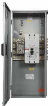
Main Circuit Breaker
