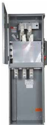
Main Fusible Switch with Utility Pull Box
