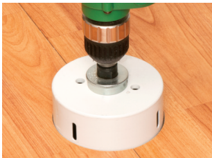
1 Using a 4" diameter hole saw, cut opening in floor approximately 1/2" deep, taking care to avoid structural framing members.
