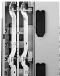
One-Piece Vertical Busbar
