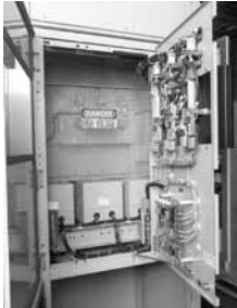
Mark V Field Controller
