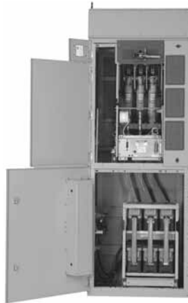
AMPGARD IT. Soft Start (Doors Open)
