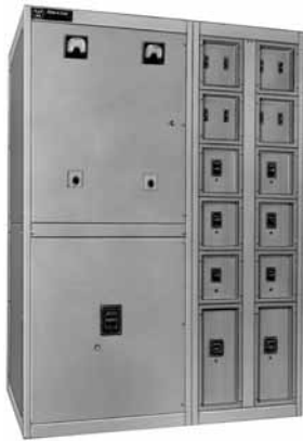
WRI Switchboard, St. Louis Vintage with Fixed Molded-Case Breakers Pow-R-I is of similar look)
