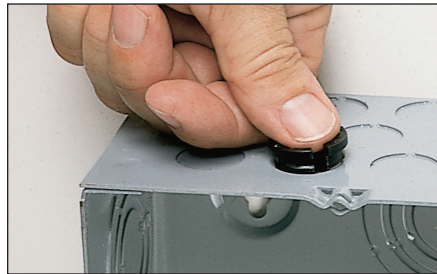
1 Push the NM cable connector into the knockout with light finger pressure.
